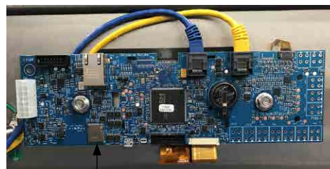
SD Card Slot on the Display Board Display Board Located on the Electrical Panel Door
